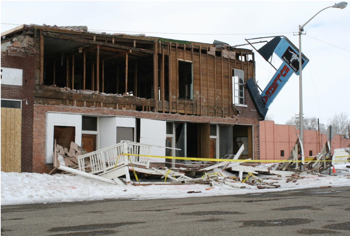
Unreinforced masonry building after Wells, NV earthquake
